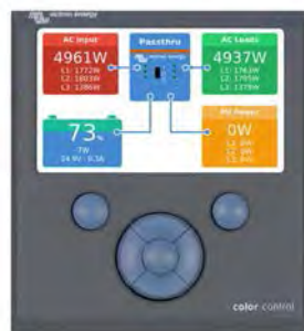
Color Control panel, showing a PV application
